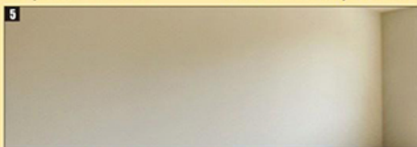
5 Allow, OSMOPLAST layer to dry for 4-6 days and now wall is ready to receive water/Cement base Paint
