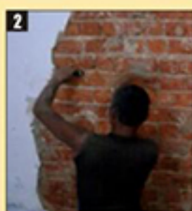
2 Expose brick work Wherever Damped spots are found by removing entire plaster layer & allow bricks to get dry for 2-3 days
