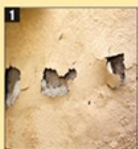
1 Excessive wall / Paint Deterioration due to prolong Dampness
